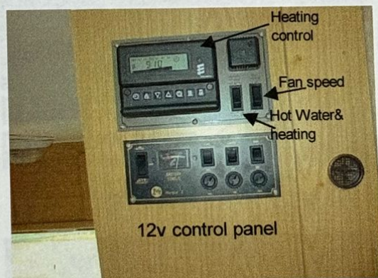
6 View showing control panels
